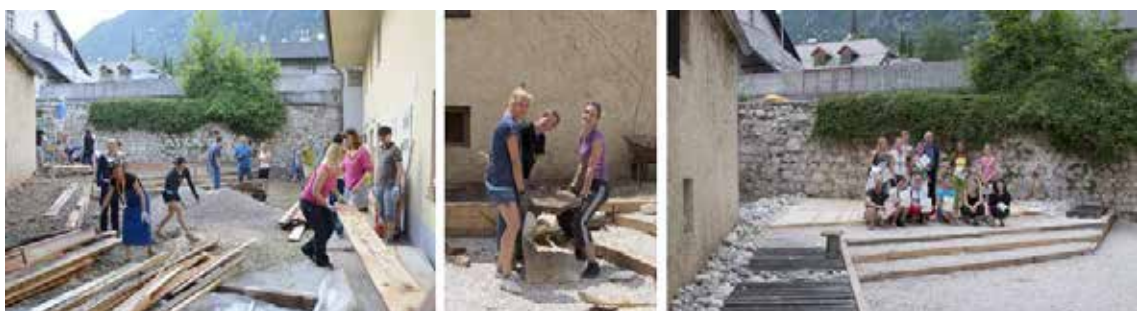
Fig. 5.25: The renovation of the courtyard with the help of 96 volunteers – building a space
