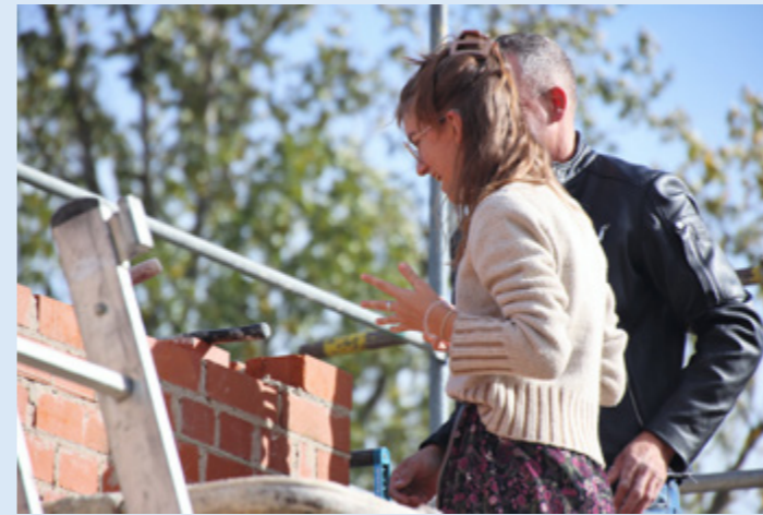
● Students tried out sustainable building techniques to safeguard the authentic quality of Herrnhut for the future.
